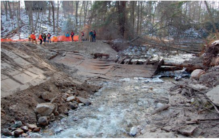
FIGURE 3. General view of fully excavated Timber Dam, north bank of brook looking southwest.
